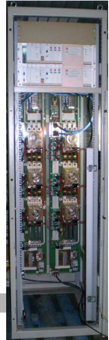
600 A energy extraction system.
