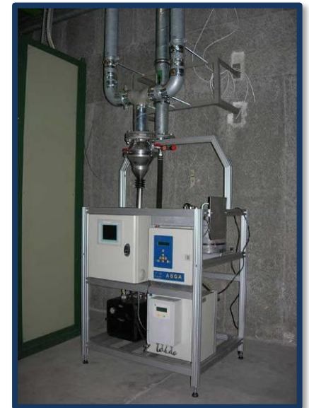
Ventilation Monitoring Stations
