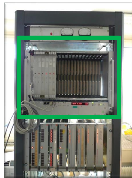
BE/CO standards for control electronics and control software
