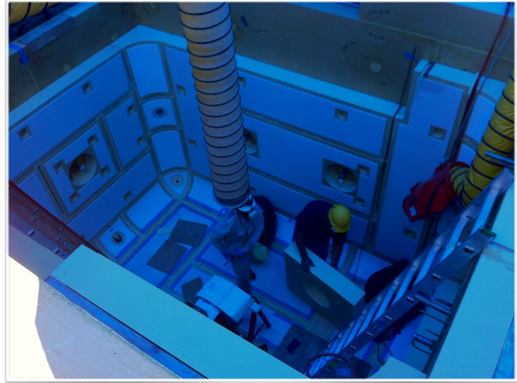
The interior of the 35 ton prototype membrane cryostat during construction at Fermilab
