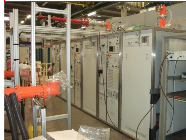
New 800 MHz IOT transmitters
