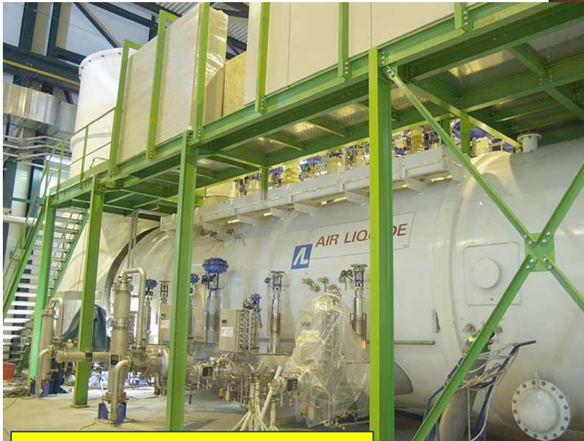
Air Liquide cold box
