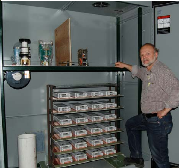
HV cabinet, Thyatron Capacitors
