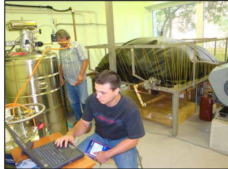
The LHeP18 (Cryomec) liquid He plant and part of the He gas recovery system
