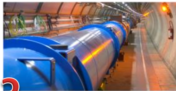
Continuous magnet line installed in the 27 km LHC tunnel, 2006
