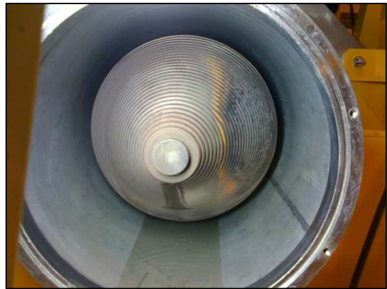
Figure 5: Klystron collector showing traces of overheating (2010).
