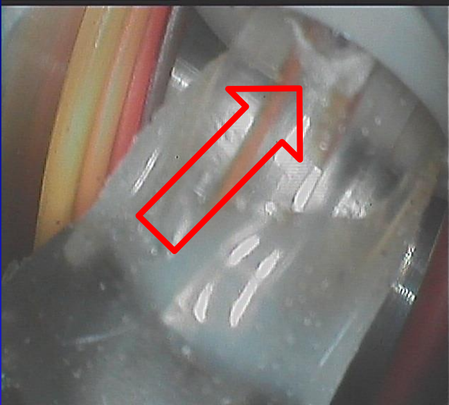
1) Inlet with little crack
