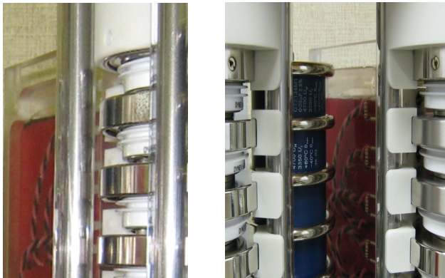
Figure 11: GTO stacks before LS1 (left) and after LS1 (right) with additional high-voltage insulation.
