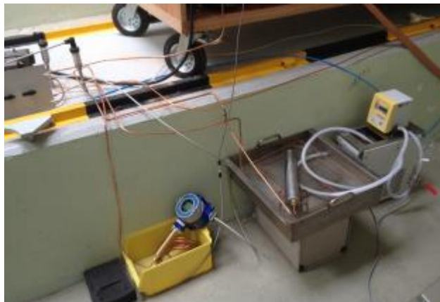
Hydrogen production measurement device
