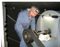
Amplifier and building coolers are not so efficient
