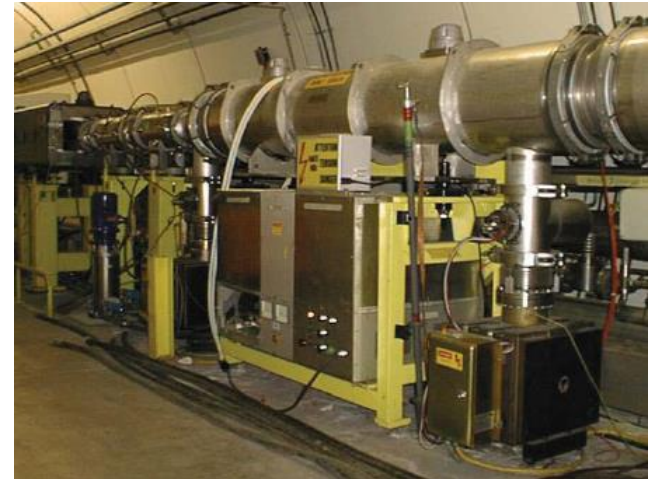
Tunnel with kicker tank and tetrode amplifier in SPS LSS2
