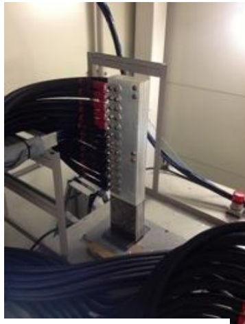
New 15kA bus lines
