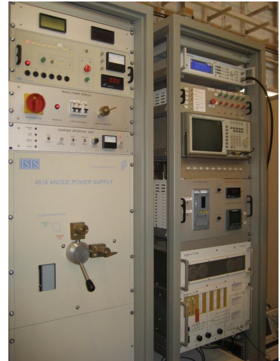
20 kV Power Supply & Aux. Rack
