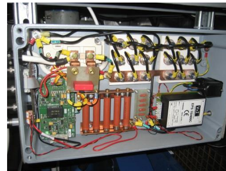
Cathode Modulator: TH116 Tube On/Off Control
