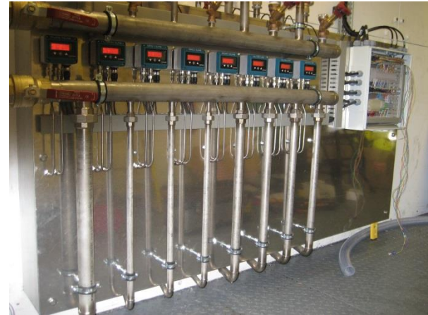
Water panel for RF in MICE Hall
