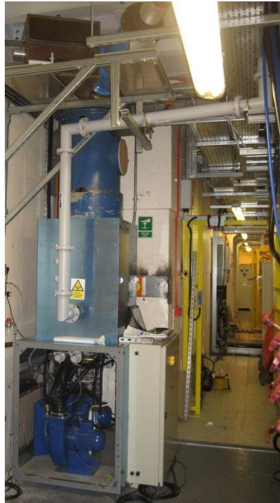
TH116 Amplifier installed in MICE Hall at RAL
