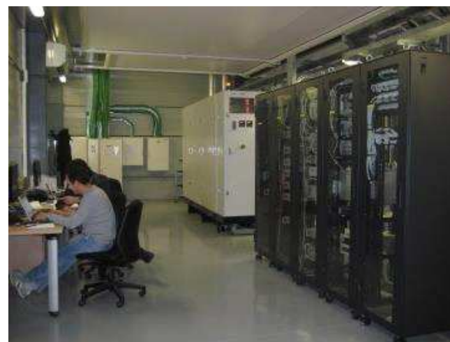
LLRF and Controls racks
