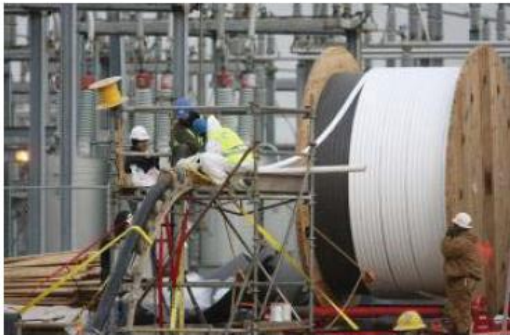
Photo courtesy of Southwire
