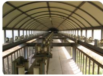
TF, PF, CC & Feeder Jacketing at ASIPP
