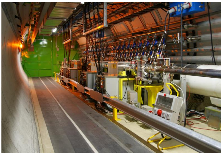
LHC transverse Feedback (ADT) kickers and amplifiers in tunnel point 4 of LHC, RB44 and RB46
