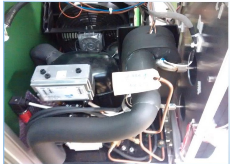
R404 Chiller inside
