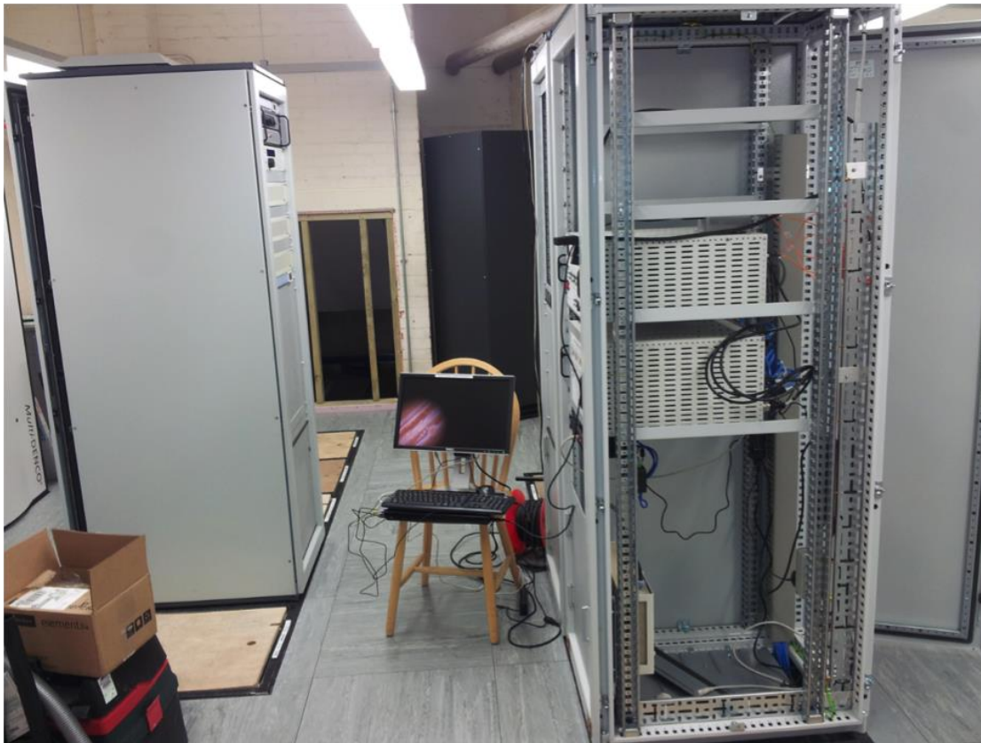
Step IV control racks
