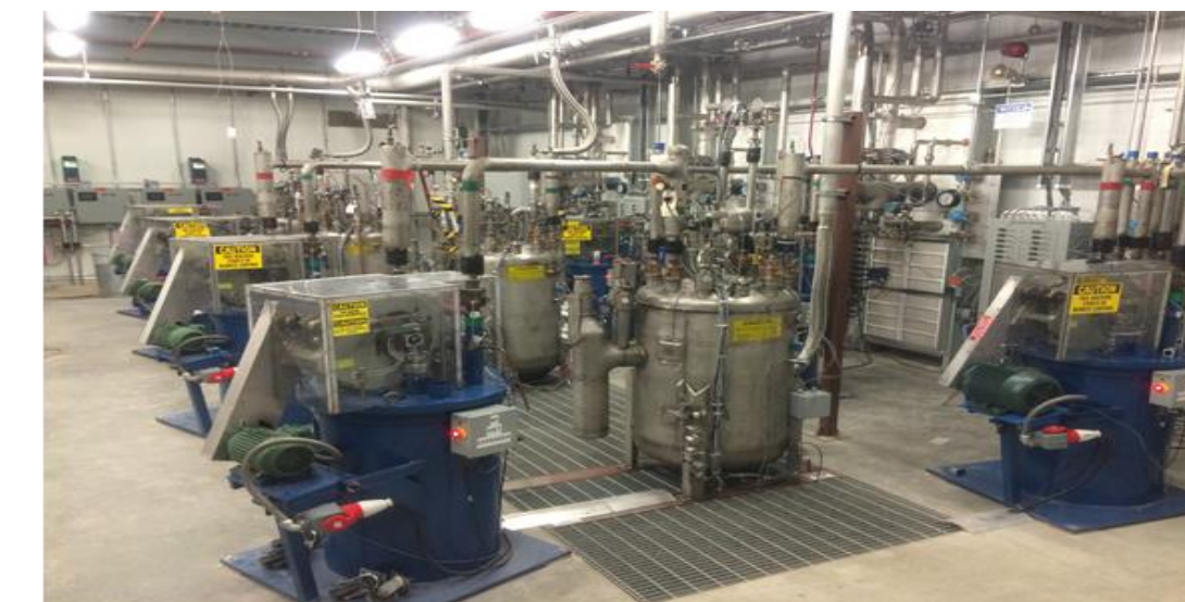
Figure 3. CM1 Four Tevatron style satellite refrigerators
