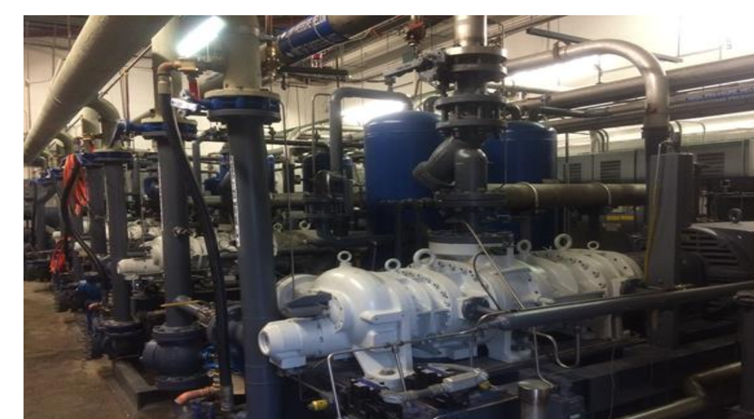
Figure 2. A0 Warm Compressor Room
