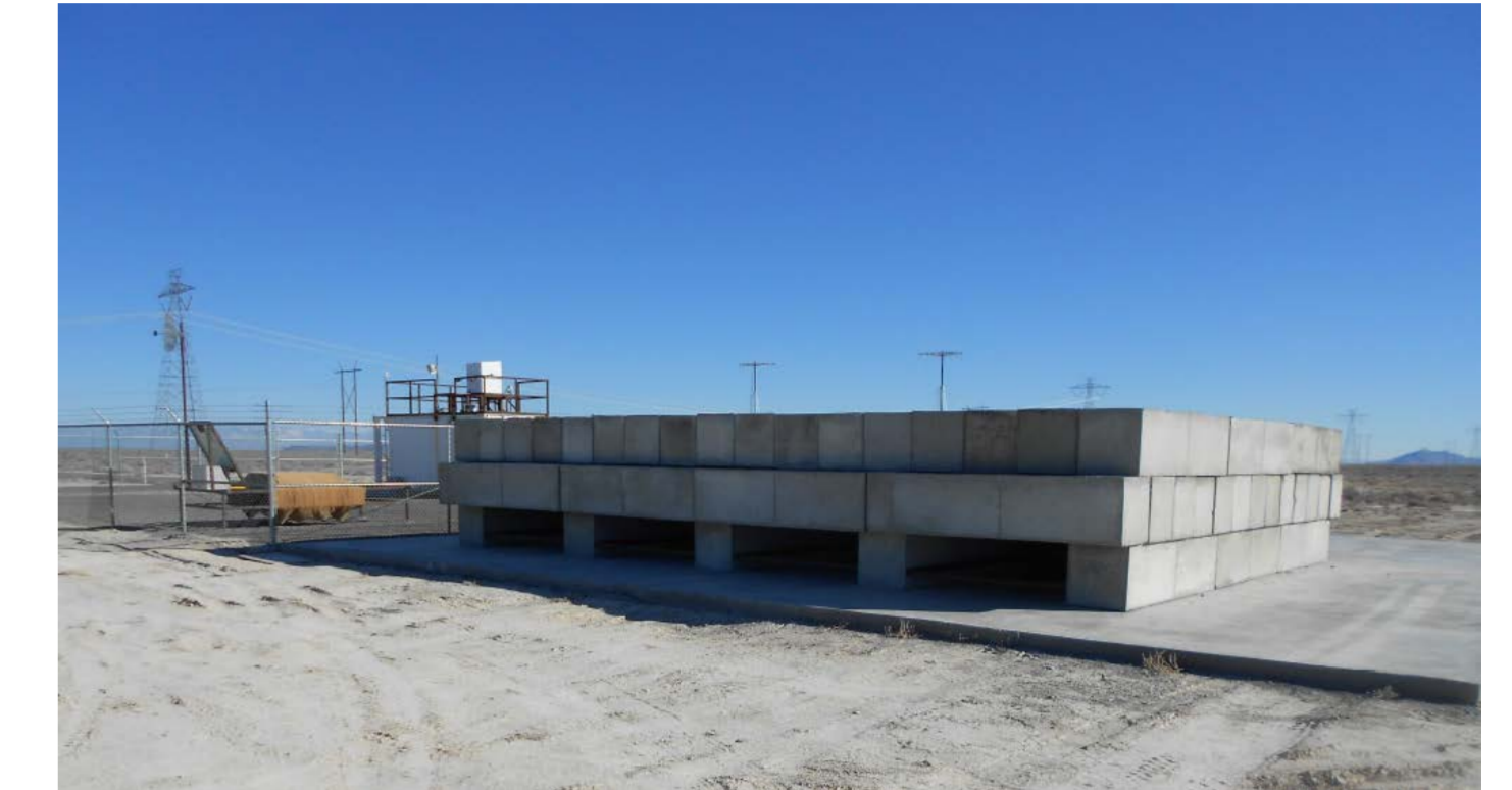
Fig. 3: Constructed concrete shield. 8 of 3m 2 detector will be inserted under the shield.
