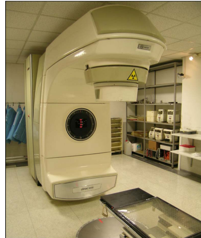
Varian Clinac 1800 installed in the S. Anna Hospital in Como (Italy)
