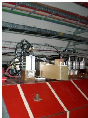
BRAN installed in TAN alongside ZDC detectors on 56 side of Pt5
