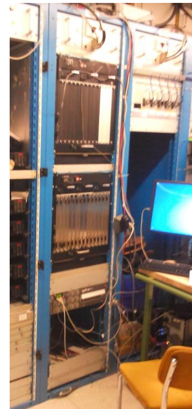
Rack in USA15
