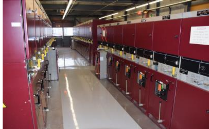
LHC8_18 KV substation
