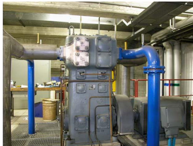
Main He compressor
