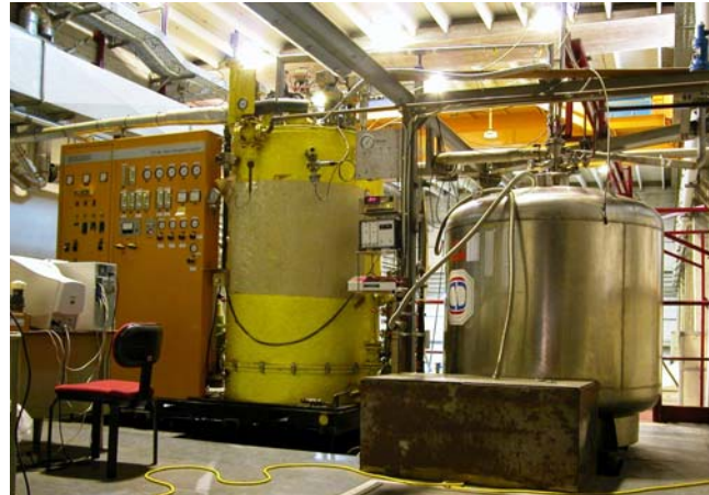
40 l/h He liquefier
