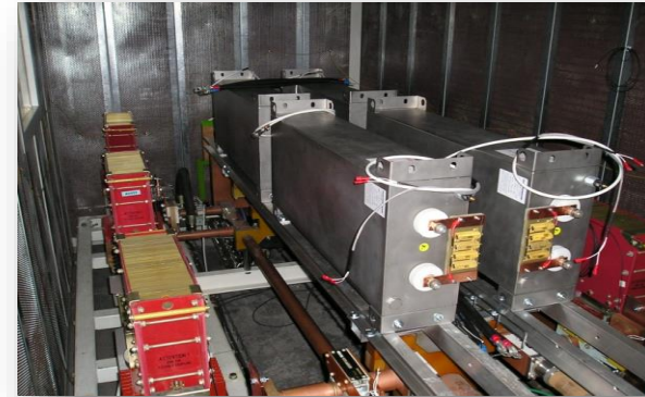
13kA EE – Snubber capacitor
