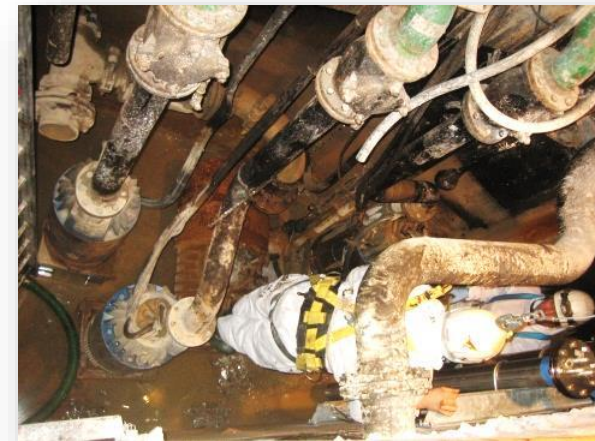
PM32 raising pumps
