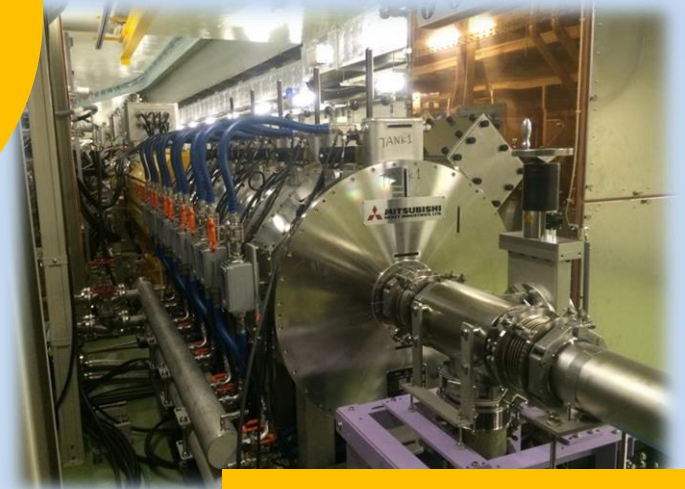
J-PARC New RF cavities
