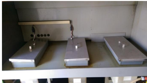
Ethylene Tank for Micro-bulks
