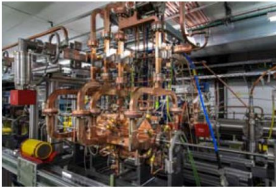
The new CLIC module in the CTF3 test facility.
