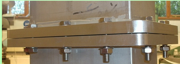
Before, loose bolts
