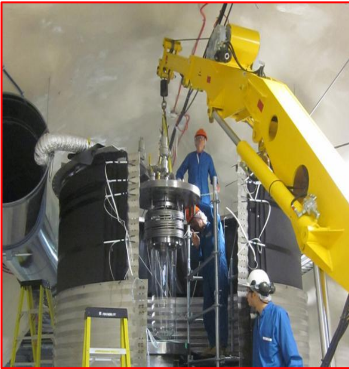
PICO-60 installation in water tank at Snolab
