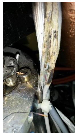
Burnt cable on DFBA
