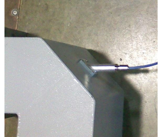
Sensor in waveguide (in Linac tunnel)
