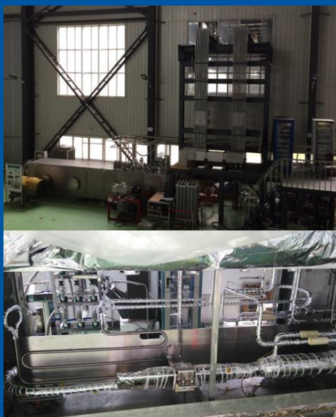
Top: Test cryostat and cubicles Bottom: Leads inside CTB
