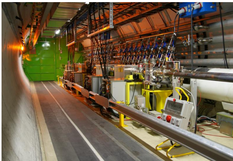
LHC transverse Feedback (ADT) kickers and amplifiers in tunnel point 4 of LHC, RB44 and RB46
