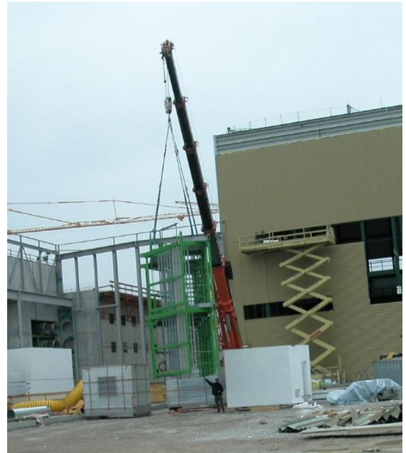
Metallic staircase in shaft for services
