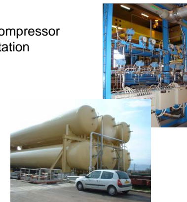
helium storage tanks
