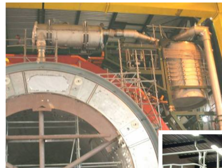
phase separator and 6000 l tank
