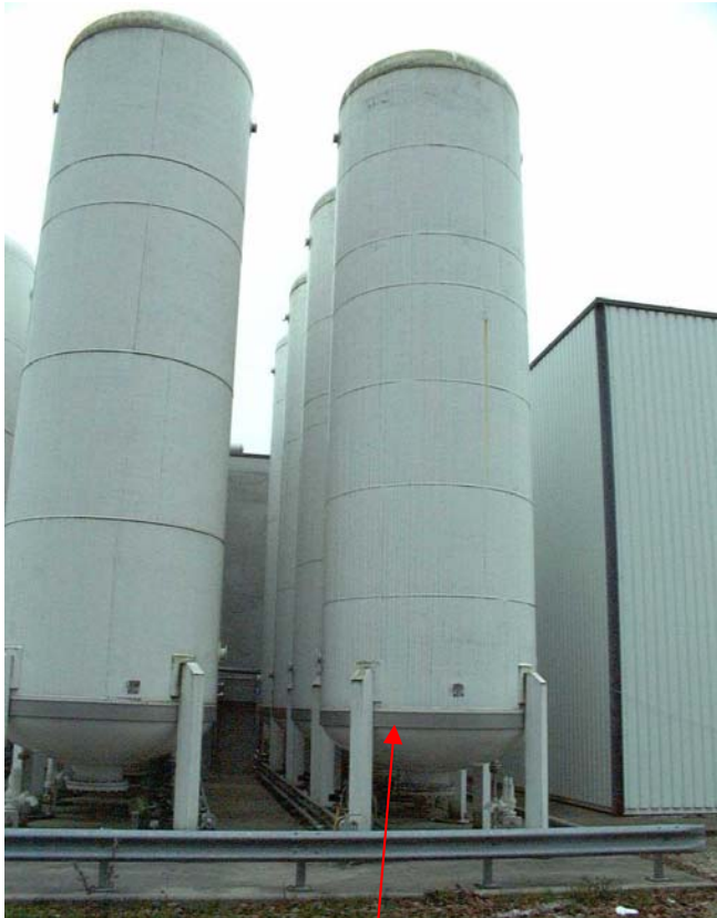
Separation of 4 former LEP2 buffers and connection to CAST cryoplant
