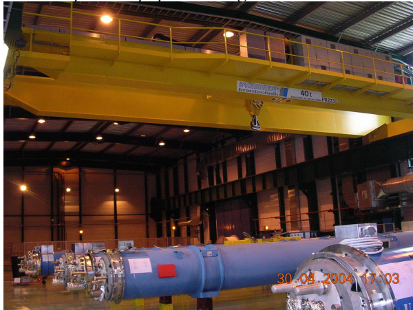
Figure 4: Brunnhuber Overhead travelling crane (40 t) in SM12
