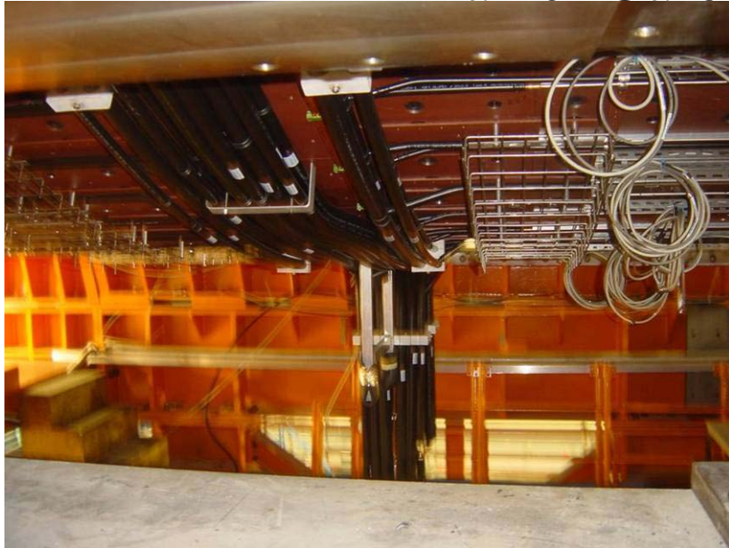
Cooling pipes, cable trays and local cables installed in the lower part
