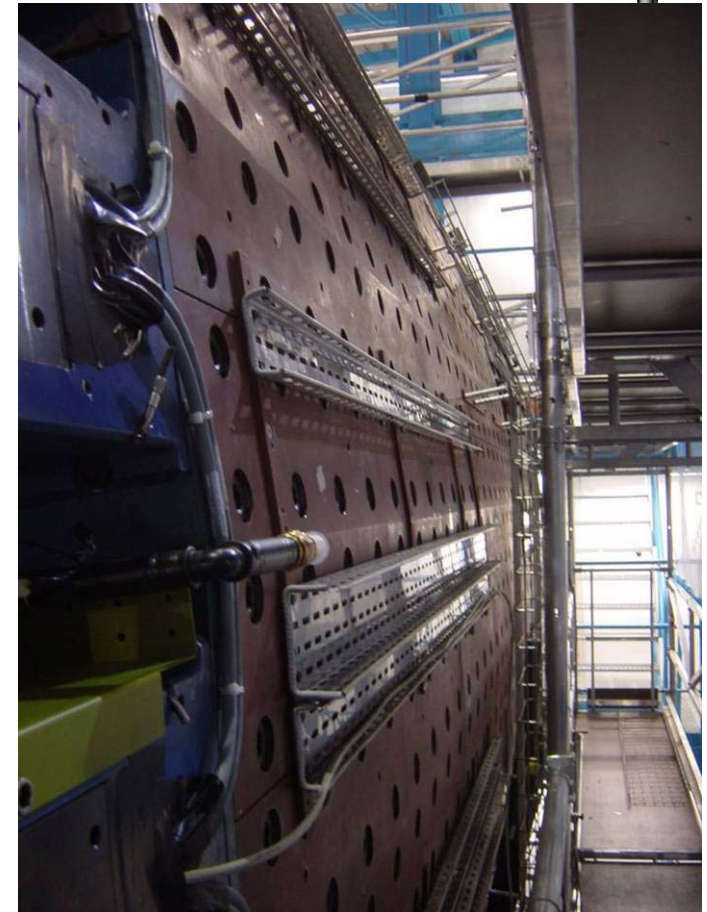
cable trays (for the calorimeters services) being installed on the rest of the cylinder
