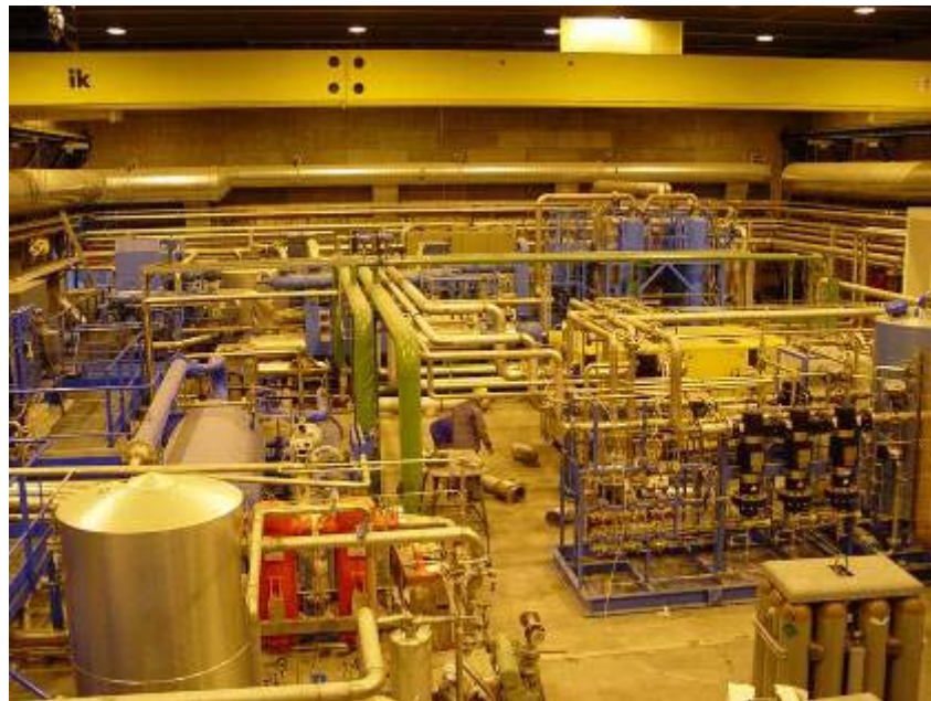
Compressor room SUX1
