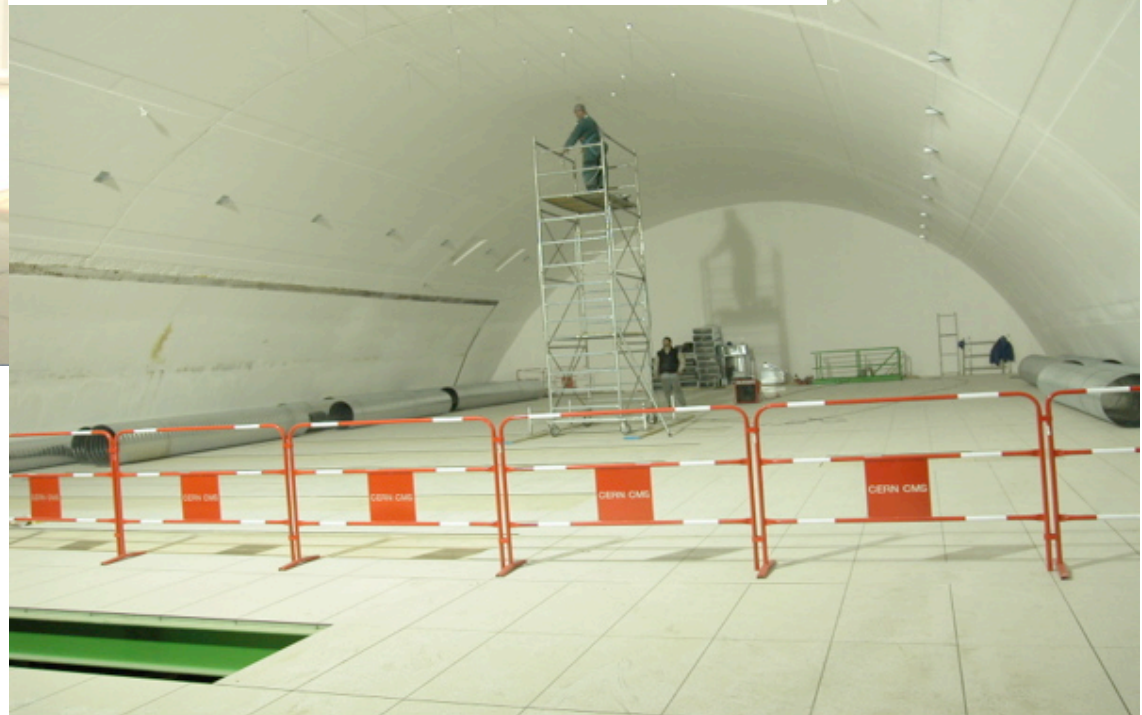
USC55- Controls First Floor
