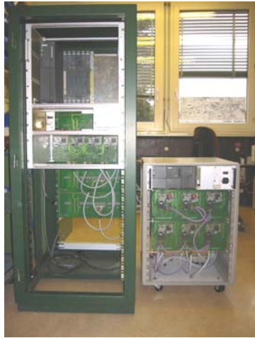
Powering Interlock Controller (PIC)
