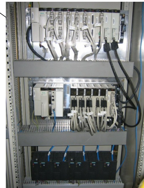
PLCs Schneider (Modicon) DP/PA couplers and links (Siemens)
