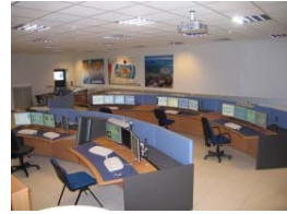
Atlas Control Room
