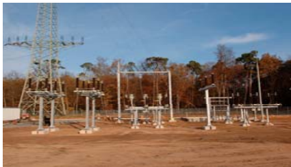
Power grid connection
