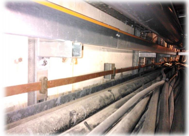
25mm x 3mm Busbar in main trench
