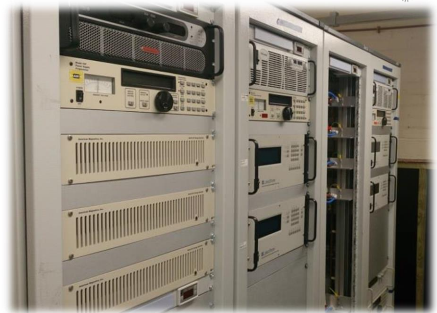
Racks installed in RR2
