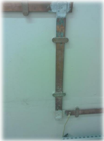
50mm x 6mm Busbar North, South & West walls
