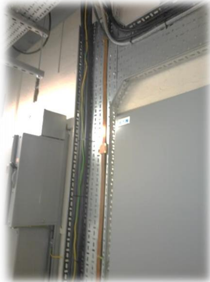
25mm x 3mm Busbar NE corner
